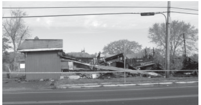
The remains of the New Gretna House the morning after the fire.
