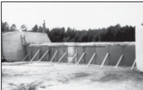
The dam, completed in 1941 by the CCC, restricted the water flow of the West Branch of the Bass River, creating Lake Absegami. (Photo courtesy of Bass River State Forest photo archives.)
